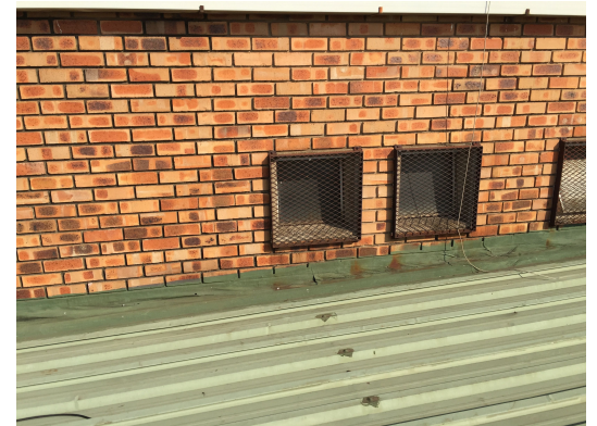
Failed metal flashing with waterproofing
